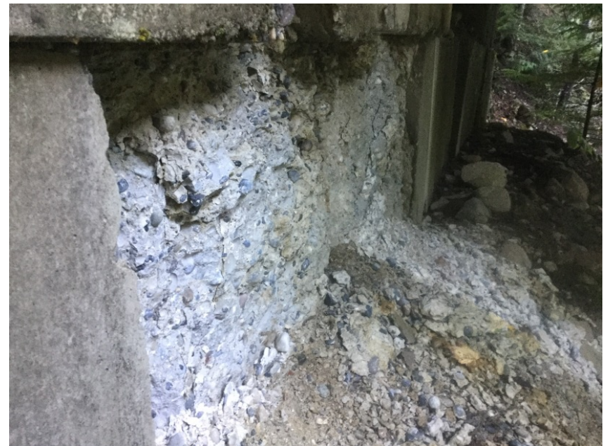
Lock block condition at right bank
